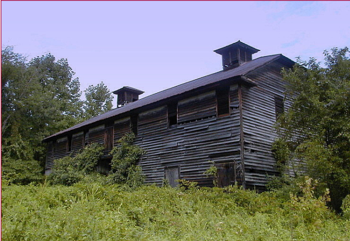
74A-014 Seton Belt Barn at Oatland Church Road (north of MD 214) Mitchellville
